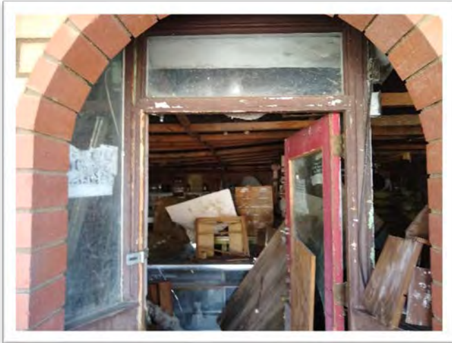
Sample 20-045A.L1, Brown Paint, 11,000 ppm Lead
