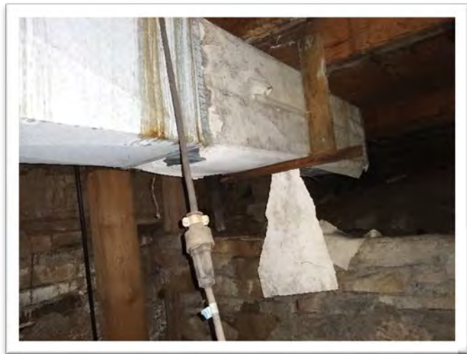
Sample 20-045A.42, Duct Insulation, 40% Asbestos
