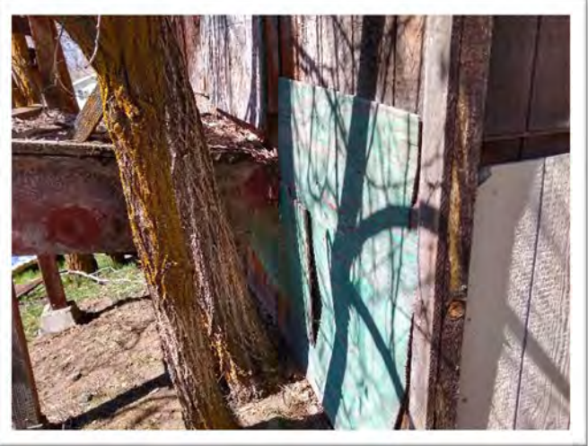
Sample 20-045A.L2, Green Paint, <64 ppm Lead
