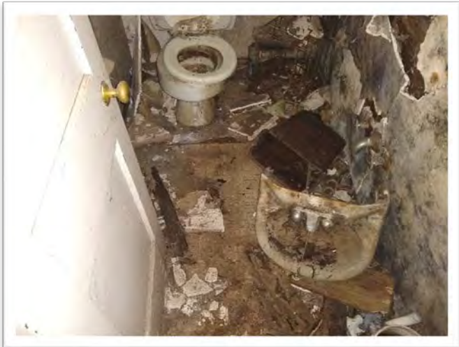
Sample 20-045A.3, Vinyl Floor, 20% Asbestos Sample 20-045A.4, Vinyl Floor, 20% Asbestos
