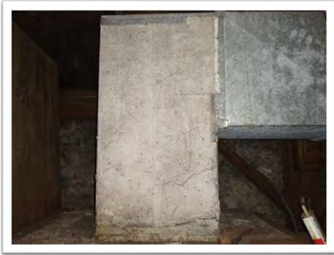
Sample 20-045A.41, Duct Insulation, 40% Asbestos
